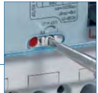
Thermal-magnetic MCCBs are adjusted on the front panel using a screwdriver
